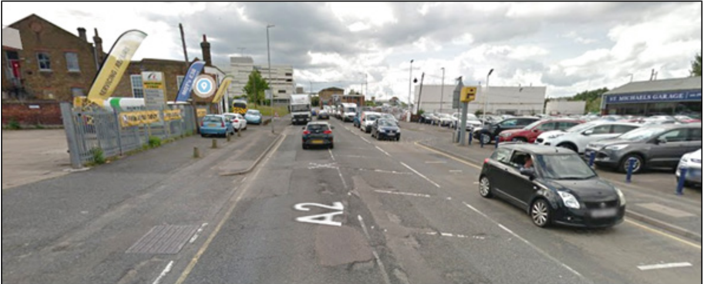
The poor condition of St Michael's Road
